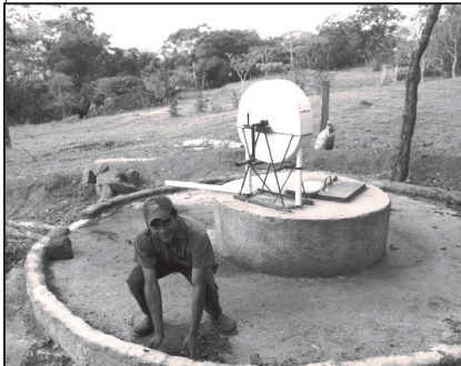
Putting the finishing touches on the well skirt, Cerro de la Cruz.
